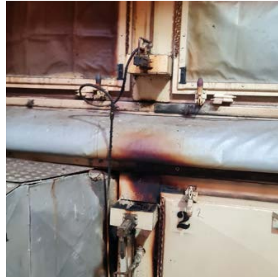
Slika 48. Instalirani platneni kompenzator/ Installed fabric expansion joint
